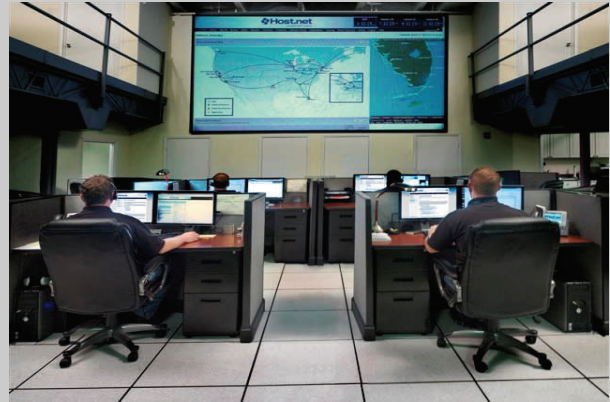
This photo was taken in Host.net’s Phase III collocation facility at their headquarters in Boca Raton, Florida
